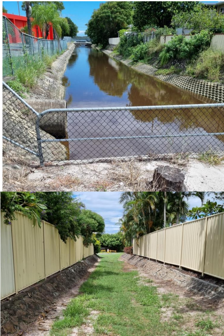
Figure 3-1 Open channel and overland flow path near Indra Ave observed on site visit, 7 th March 2022
