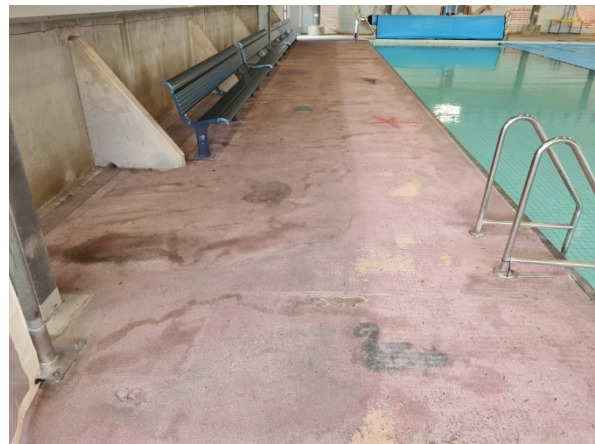
Figure 3: Image of Deteriorated Artwork (18.3m Pool)
