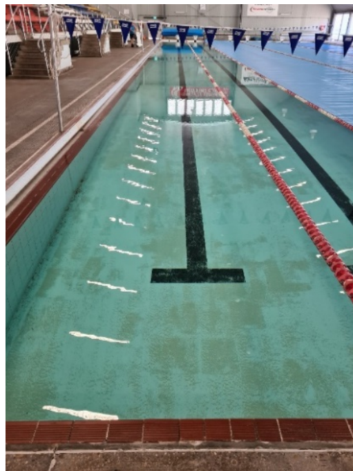
Figure 1: Image of 50m Pool Deterioration
