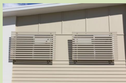
(Maroochydore) Fixed screening over windows is not a desirable solution to overlooking as shown above. Windows should be offset or have an appropriate separation distance.
